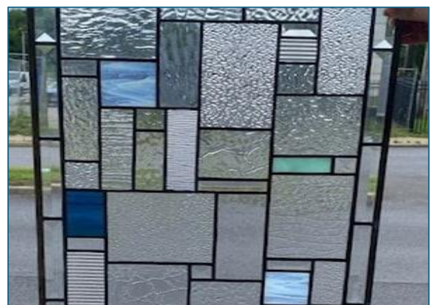
Figure 1: Multiple stained pieces in the window glass.
