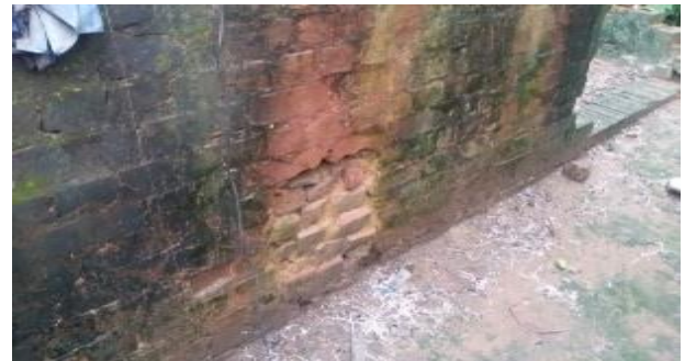
Figure 2: Temporary door bricked up after use.
